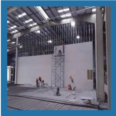
Fire Rated Drywall Partition
