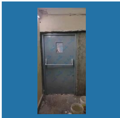
Fire Rated Shaft Doors
